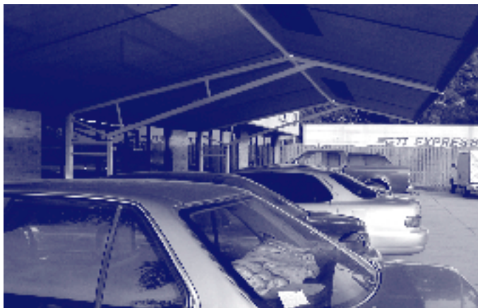
Sunguard Shade Structures Sarasota, FL
