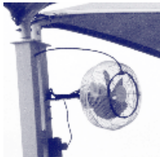
Lackland Air Force Base Misting System San Antonio, TX
